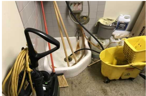
#30 FLOOR SERVICE SINK
