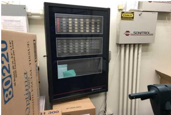
#47 FIRE CONTROL PANEL
