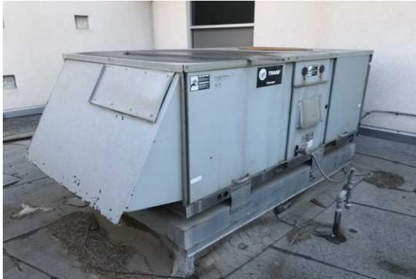
#37 ROOF TOP PACKING UNIT
