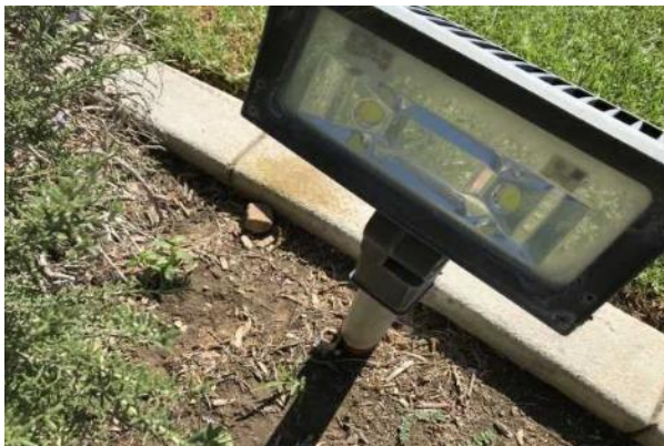
#45 LED EXTERIOR BUILDING LIGHT
