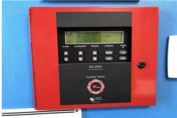
#49 ANNUNCIATOR ALARM PANEL
