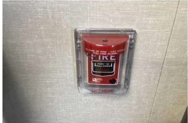
#50 FIRE PULL STATION
