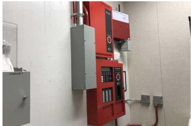
#48 FIRE CONTROL PANEL
