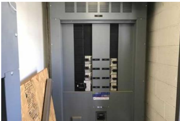
#41 INTERIOR ELECTRICAL PANEL
