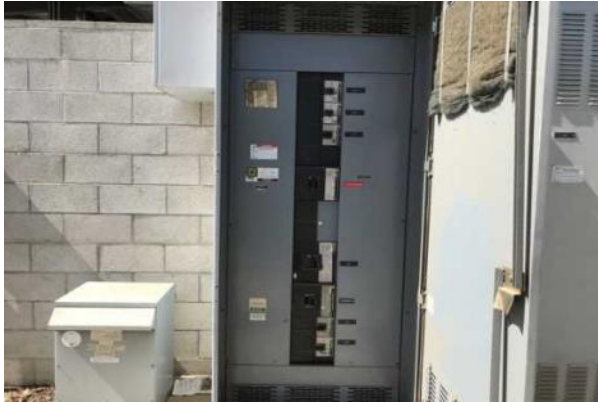
#43 EXTERIOR ELECTRICAL PANEL
