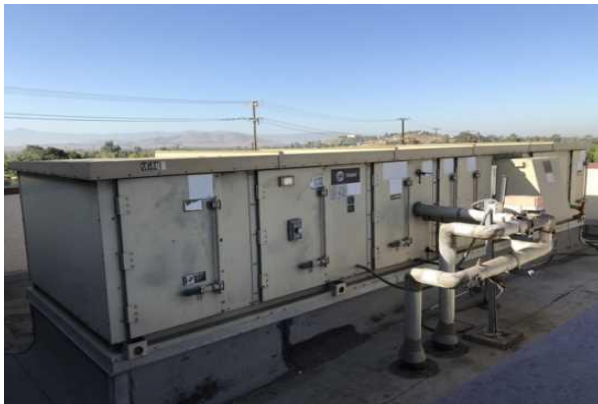
#35 ROOFTOP AIR HANDLER
