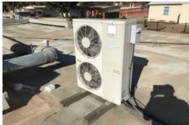
#24 DUCTLESS SPLIT SYSTEM
