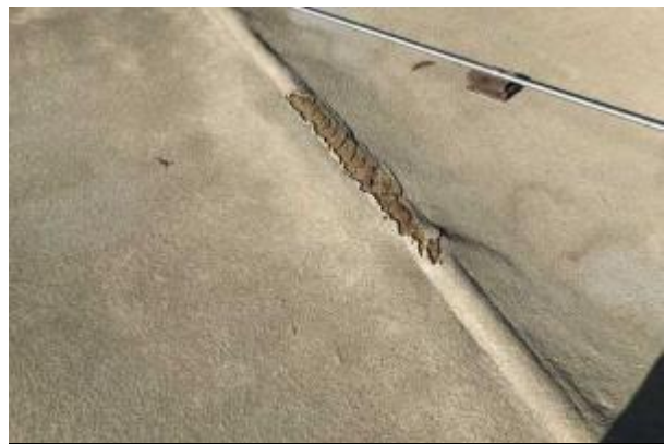
#10 BUILT-UP ROOFING, PEELING AND CRACKING
