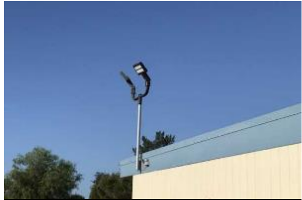
#26 EXTERIOR BUILDING LED LIGHTING
