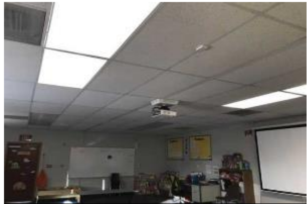
#28 INTERIOR LIGHTING SYSTEM
