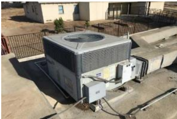
#23 ROOFTOP PACKAGE UNIT
