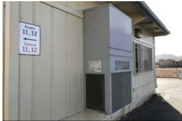
#22 WALL MOUNTED HEAT PUMP
