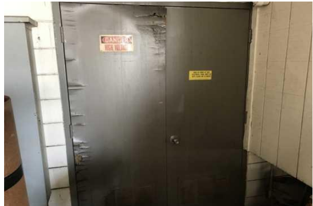
#40 DAMAGED DOORS TO UTILITY CLOSET
