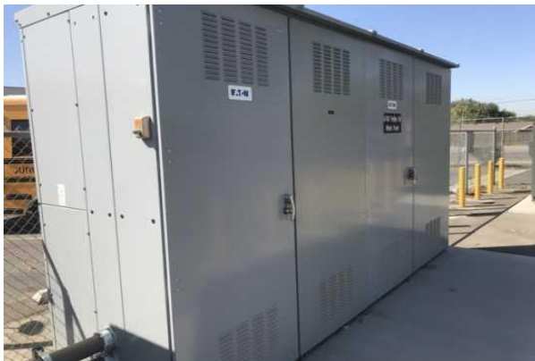
#27 MAIN ELECTRICAL EQUIPMENT
