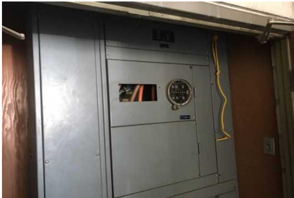
#39 ANTIQUATED ELECTRICAL INFRASTRUCTURE
