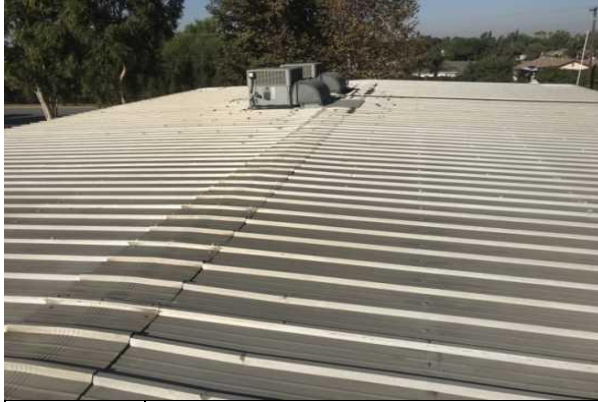
#43 PRINT SHOP ROOF LEAKS REPORTED
