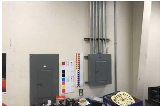
#28 SECONDARY ELECTRICAL EQUIPMENT
