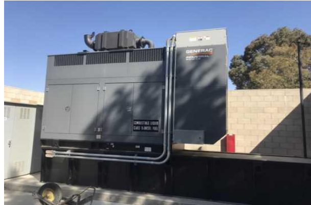
#32 EMERGENCY GENERATOR, SERVER BUILDING
