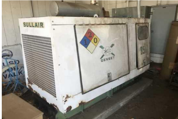
#31 EMERGENCY GENERATOR, MAIN BUILDING
