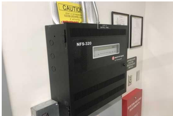
#33 FIRE ALARM CONTROL PANEL
