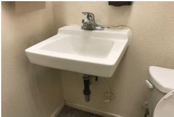
#41 LAVATORIES LACK PIPE WRAPS
