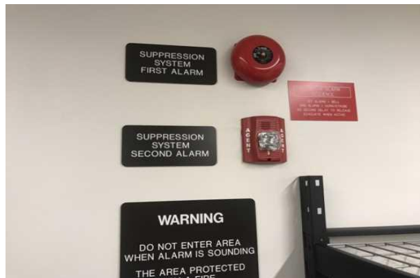
#36 FIRE SUPPRESSION SYSTEM, SERVER BUILDING
