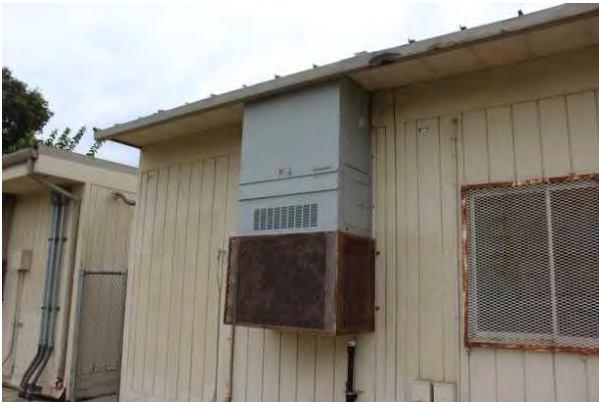
#27 HEAT PUMP, WALL-MOUNTED
