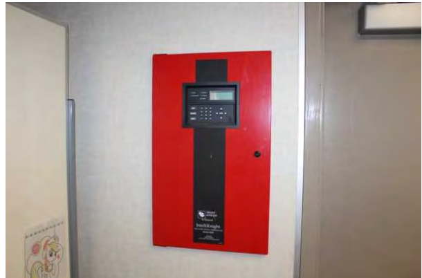
#34 FIRE ALARM CONTROL PANEL, ADDRESSABLE
