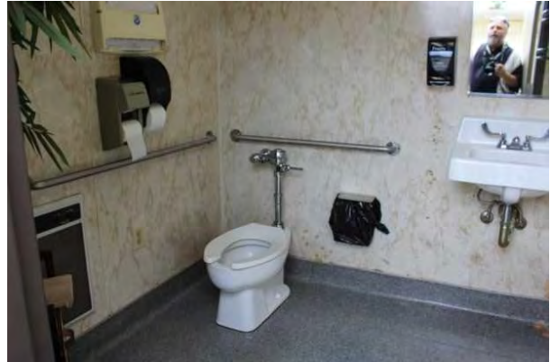
#20 TOILET, COMMERCIAL WATER CLOSET
