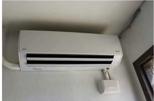
#26 DUCTLESS SPLIT SYSTEM, MULTI ZONE
