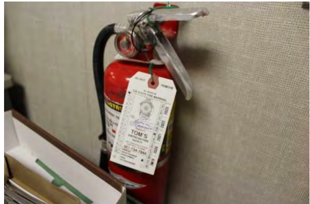
#28 FIRE EXTINGUISHER, TYPE ABC
