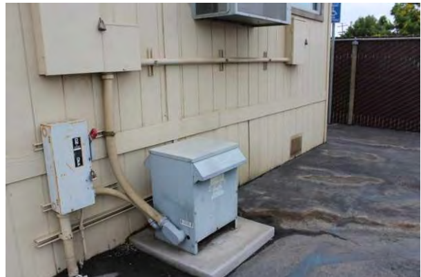
#30 SECONDARY TRANSFORMER, DRY
