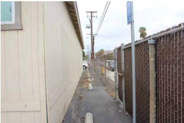
#41 FENCES AND GATES, CHAIN LINK
