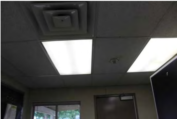
#33 LIGHTING SYSTEM, INTERIOR T8
