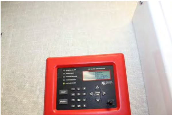
#35 ANNUNCIATOR ALARM PANEL
