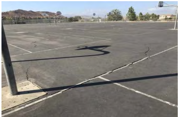
#48 DEFICIENCY - CRACKED PAVEMENT
