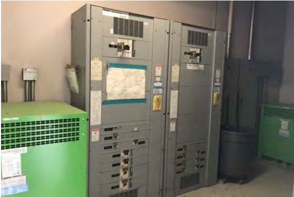
#31 BUILDING B ELECTRICAL SYSTEM
