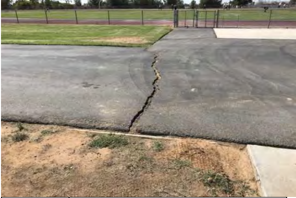
#49 DEFICIENCY - CRACKED PAVEMENT
