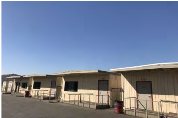
#46 DEFICIENCY - WOOD STUDS
