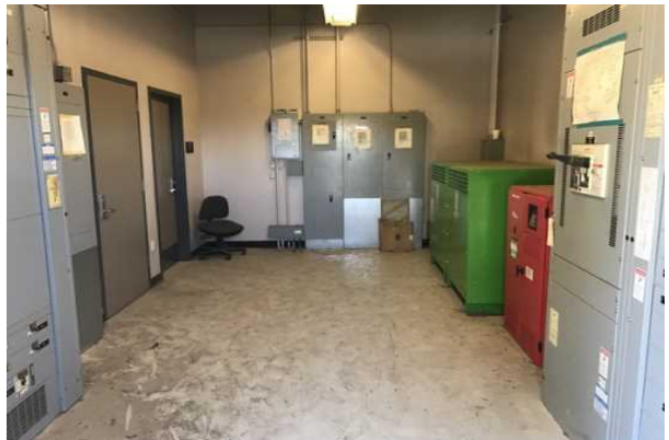
#30 BUILDING D - ELECTRICAL ROOM
