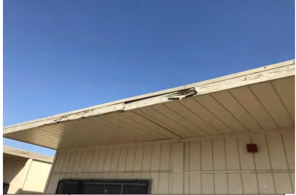
#50 DEFICIENCY - WOOD STUDS
