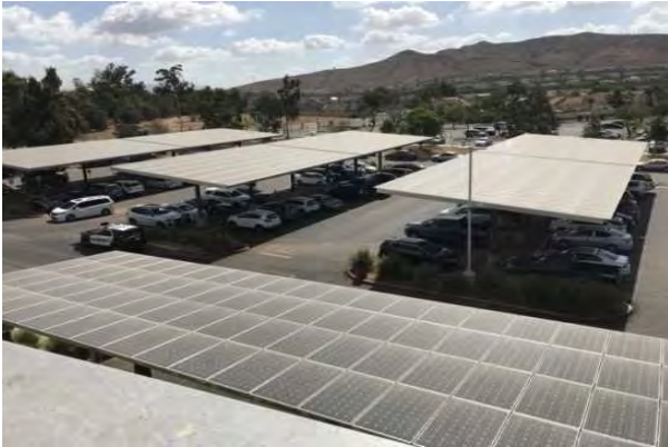
#43 CARPORTS SOLAR PANEL
