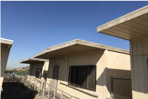
#45 DEFICIENCY - WOOD STUDS
