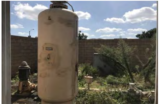
#28 CAMPUS PUMP STATION
