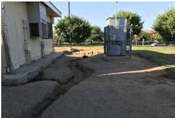
#71 PROPERTY DRAINAGE ISSUES
