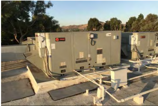
#31 ROOFTOP PACKAGE UNIT
