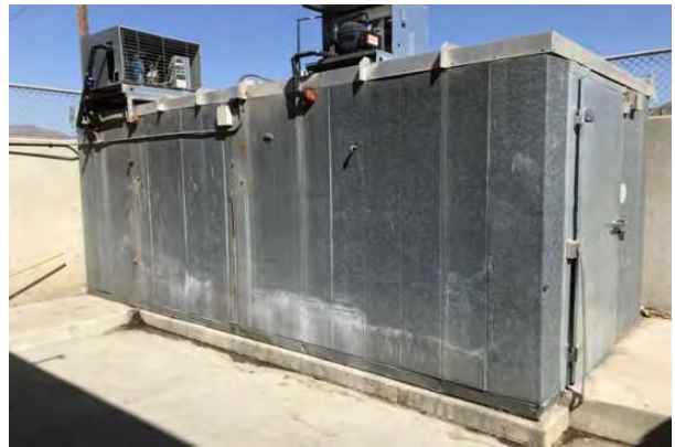
#64 EXTERIOR FREEZER/ REFRIGERATOR COMBO
