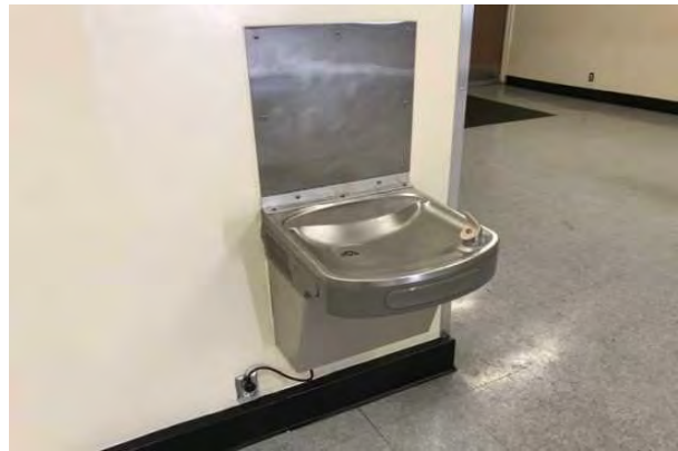
#22 INTERIOR DRINKING FOUNTAIN
