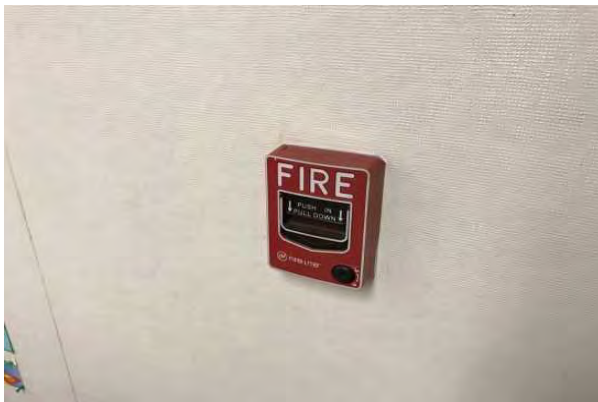
#47 FIRE PULL STATION
