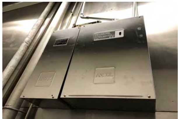
#46 KITCHEN FIRE SUPPRESSION SYSTEM
