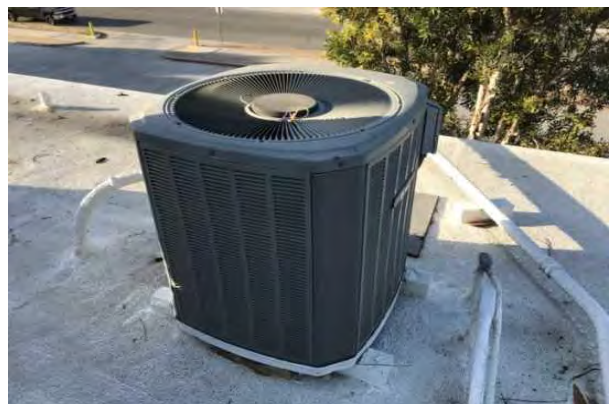
#36 ROOFTOP CONDENSING UNIT
