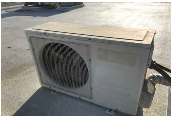
#33 DUCTLESS SPLIT SYSTEM UNIT
