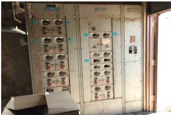
#41 EXTERIOR MAIN ELECTRICAL PANEL
