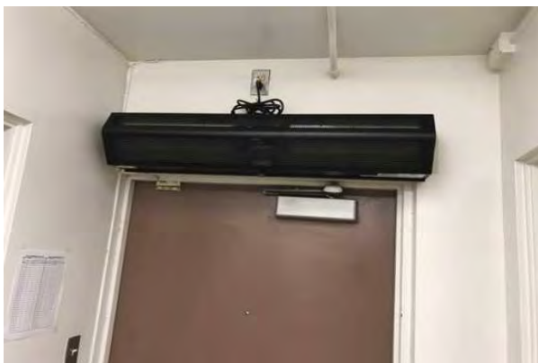
#29 AIR CURTAIN UNIT
