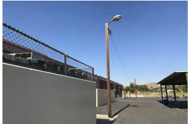
#44 EXTERIOR POLE LIGHTING
