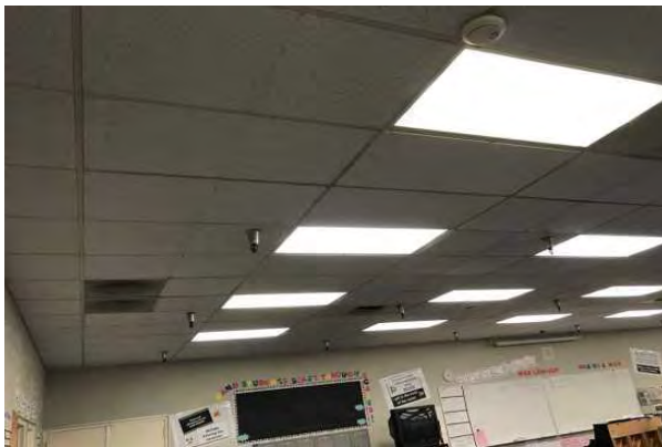
#53 INTERIOR SPRINKLER SYSTEM
