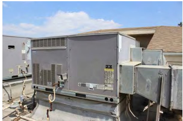
#42 PACKAGED UNIT (RTU)
