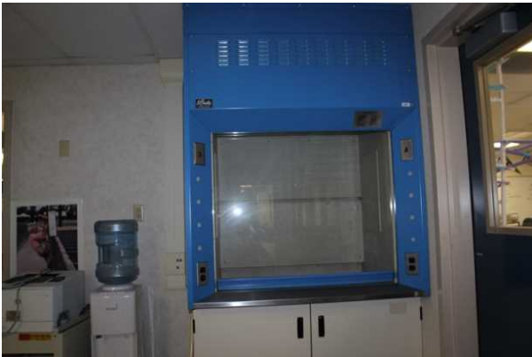
#51 LABORATORY EXHAUST HOOD
