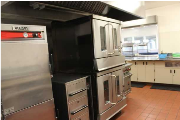
#57 COMMERCIAL KITCHEN, CONVECTION OVEN, DOUBLE
