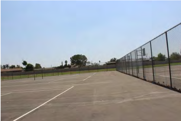
#61 FENCES AND GATES, CHAIN LINK
