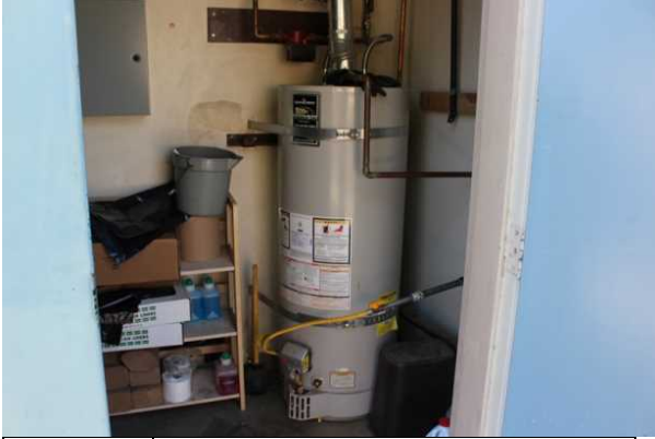
#37 WATER HEATER, GAS
