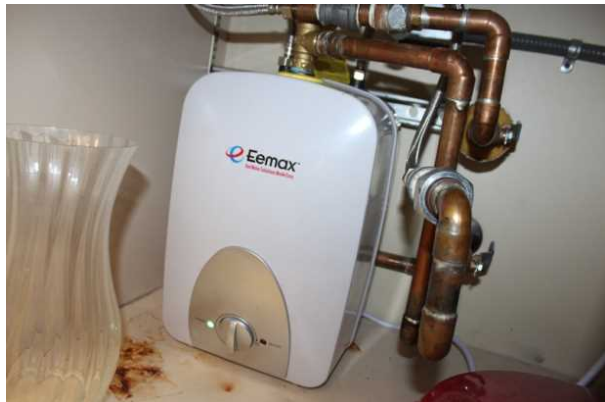
#36 WATER HEATER, INSTANT HOT
