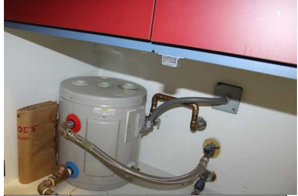
#38 WATER HEATER, ELECTRIC
