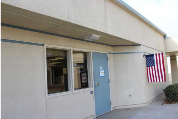
#49 LIGHT FIXTURE, EXTERIOR FLOOD
