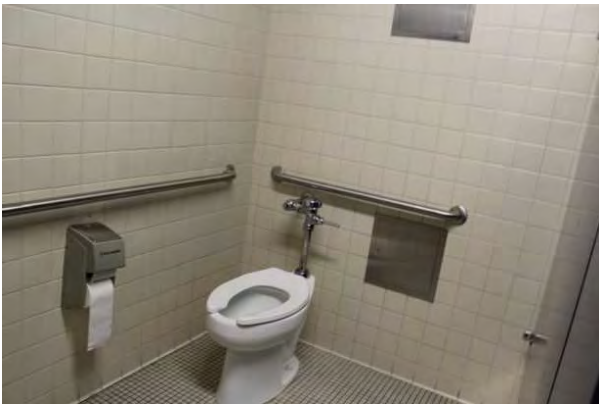
#29 TOILET, COMMERCIAL WATER CLOSET
