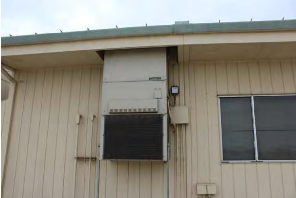
#43 HEAT PUMP, WALL-MOUNTED
