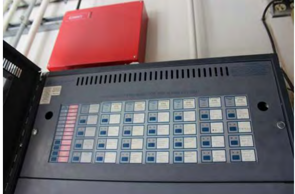
#50 FIRE ALARM CONTROL PANEL, ADDRESSABLE
