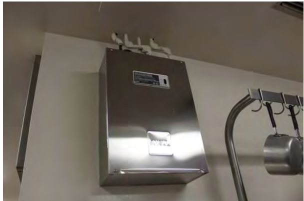
#46 FIRE SUPPRESSION SYSTEM, COMMERCIAL KITCHEN
