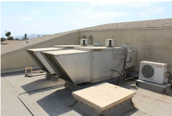
#41 MAKE-UP AIR UNIT
