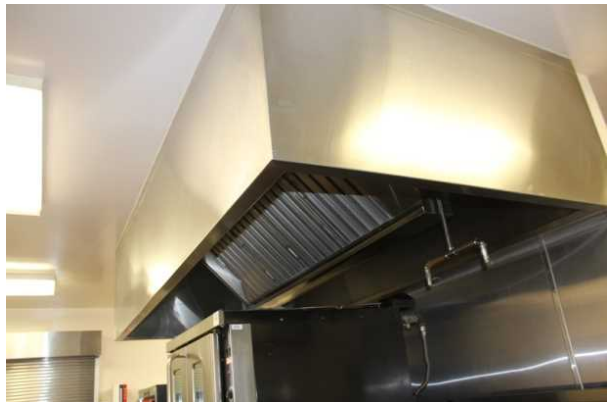
#54 COMMERCIAL KITCHEN, EXHAUST HOOD
