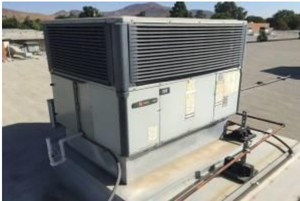
#39 PACKAGED UNIT (RTU)
