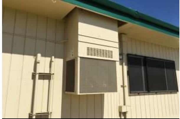
#20 PACKAGED WALL UNIT
