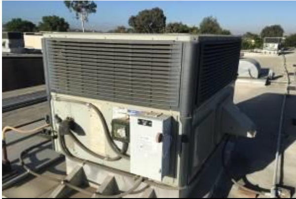
#25 PACKAGED UNIT (RTU)
