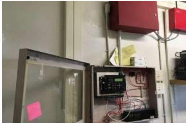
#40 FIRE ALARM CONTROL PANEL,
