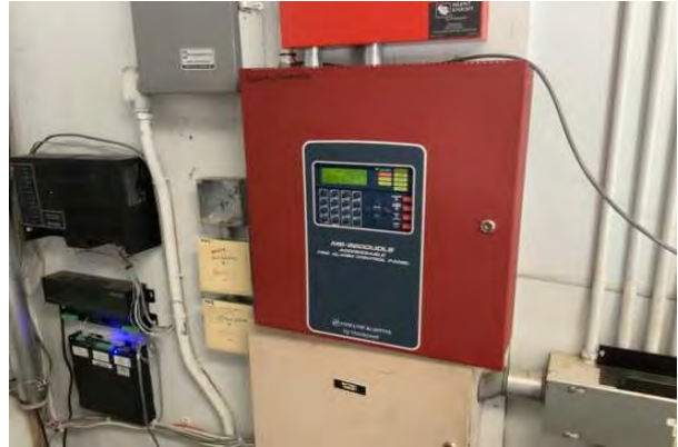
#50 FIRE ALARM PANEL
