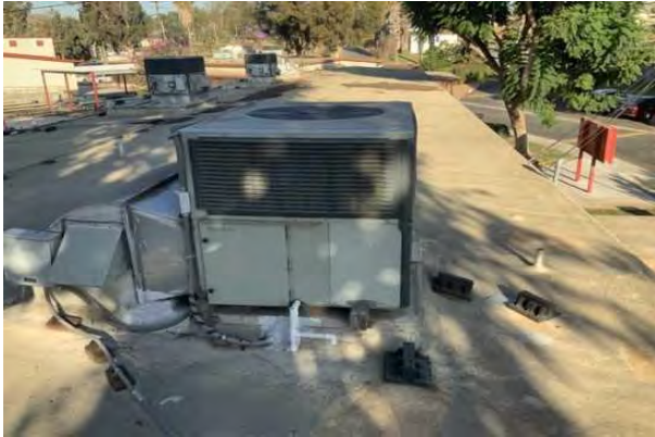
#44 PACKAGED UNIT (RTU)
