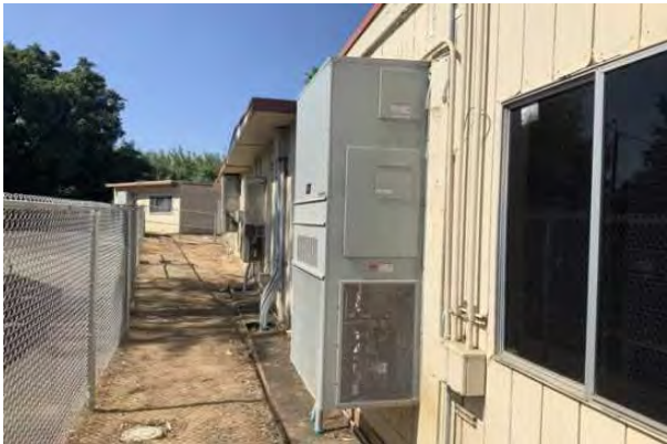
#46 HEAT PUMP, WALL-MOUNTED
