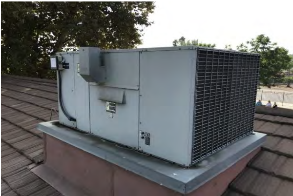
#39 BUILDING C PACKAGED UNIT (RTU)
