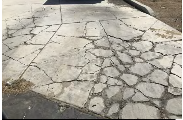
#20 DAMAGED CONCRETE FLOORING AT TRASH ENCLOSURE
