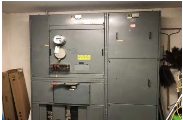
#46 BUILDING M NEW BUILDING SWITCHBOARD
