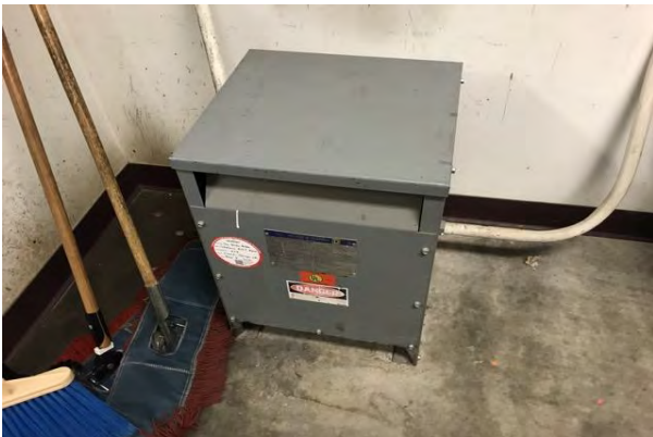
#47 BUILDING M SECONDARY TRANSFORMER
