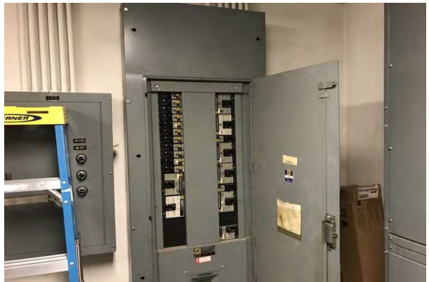
#48 BUILDING M MAIN DISTRIBUTION PANEL
