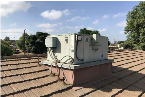
#41 BUILDING E PACKAGED UNIT (RTU)
