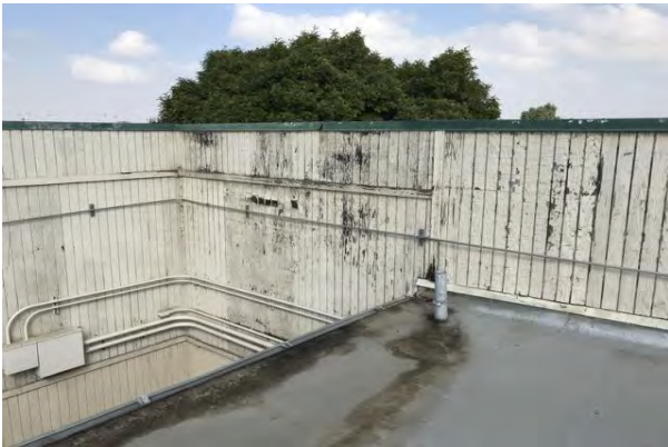
#21 DAMAGED EXTERIOR WALL AT BUILDING M
