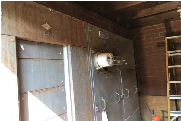
#45 MAIN ELECTRICAL ROOM OLD BUILDING SWITCHBOARD
