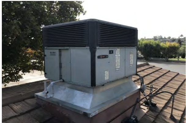
#40 BUILDING D PACKAGED UNIT (RTU)
