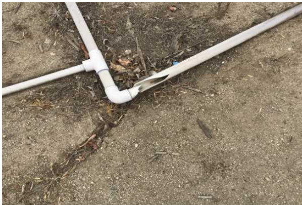
#45 EXPOSED AND RUPTURED IRRIGATION PIPING
