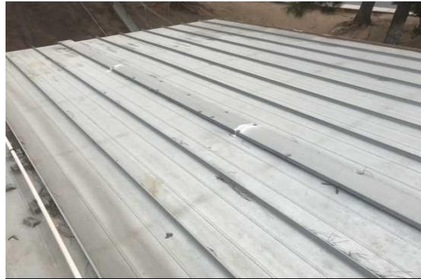
#44 PORTABLES ROOFS LEAK
