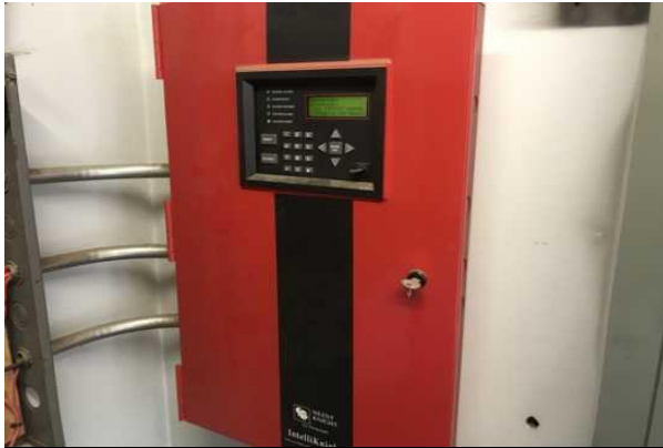
#37 FIRE ALARM CONTROL PANEL
