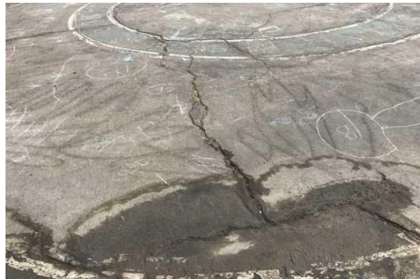
#46 PLAY/PEDESTRIAN ASPHALT CRACKING
