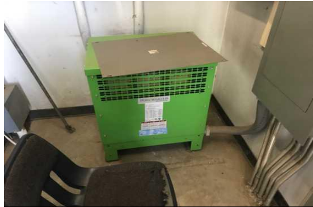
#32 SECONDARY ELECTRICAL EQUIPMENT
