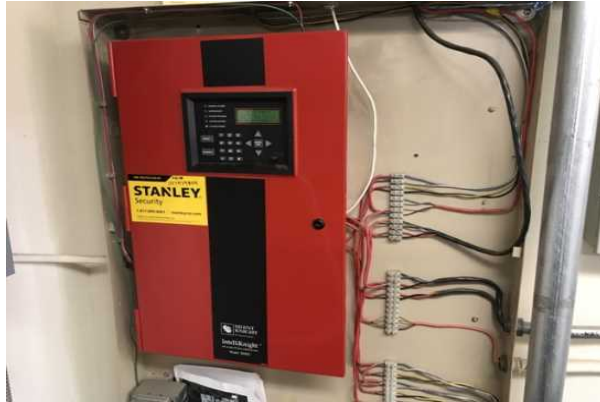
#37 FIRE ALARM CONTROL PANEL
