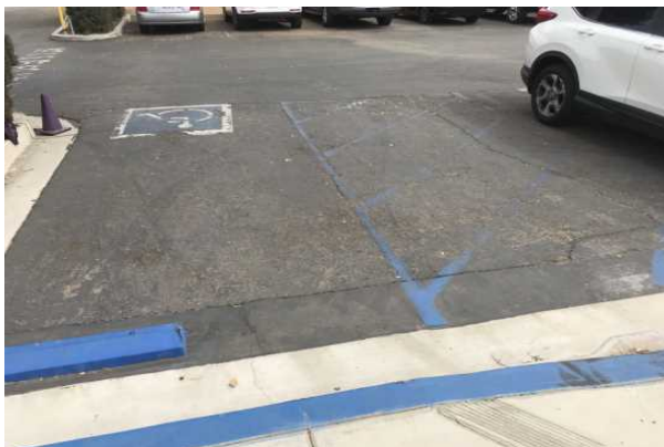
#47 WORN STRIPING, DEGRADED SEALCOAT
