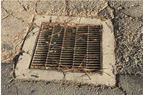
#43 INSUFFICIENT SITE DRAINAGE
