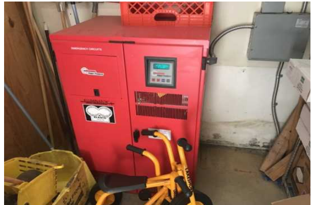
#34 UNINTERRUPTIBLE POWER SUPPLY (UPS)
