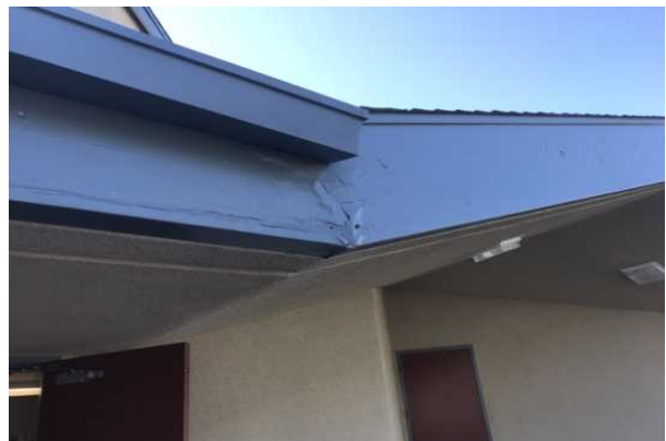
#48 ROOF TRIM ISSUE
