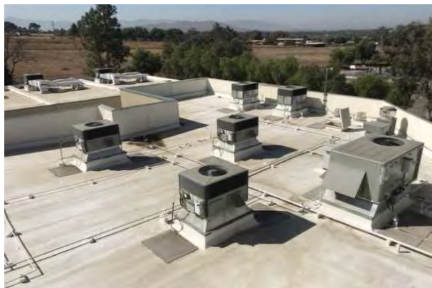
#30 COOLING MAIN COMPONENTS
