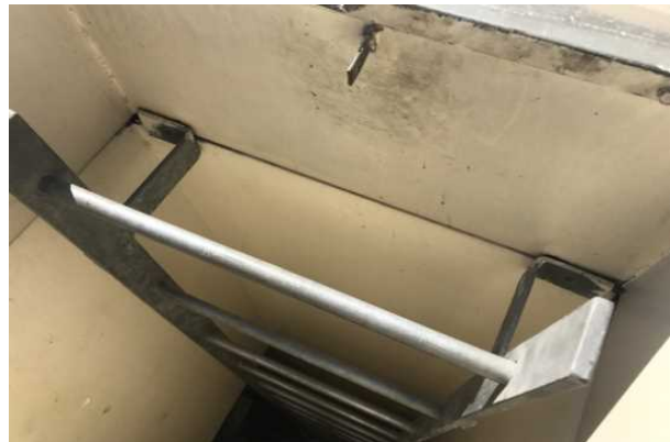
#42 ROOF HATCH ISSUE
