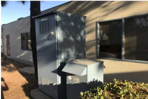
#33 SECONDARY ELECTRICAL EQUIPMENT
