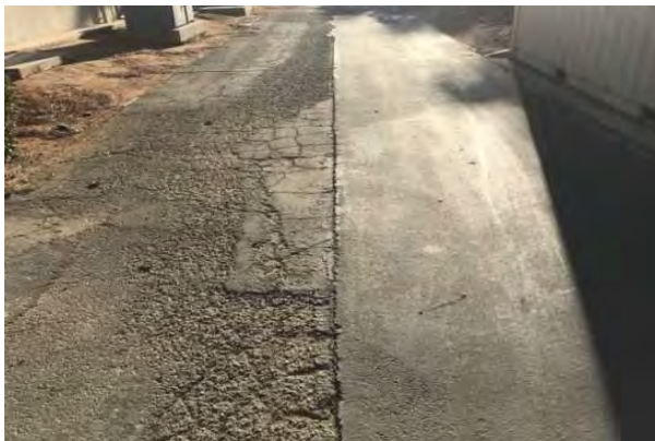
#45 DAMAGED ASPHALT PAVEMENT
