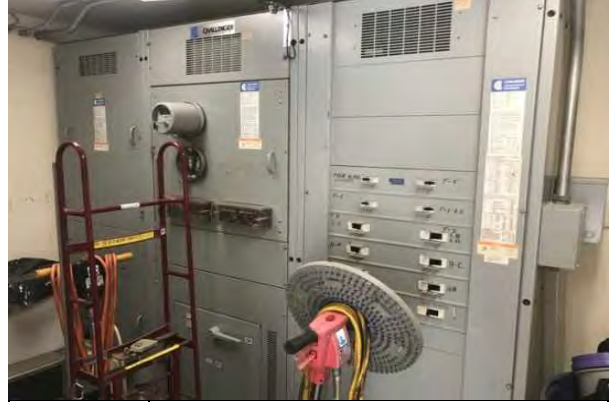
#32 MAIN ELECTRICAL EQUIPMENT
