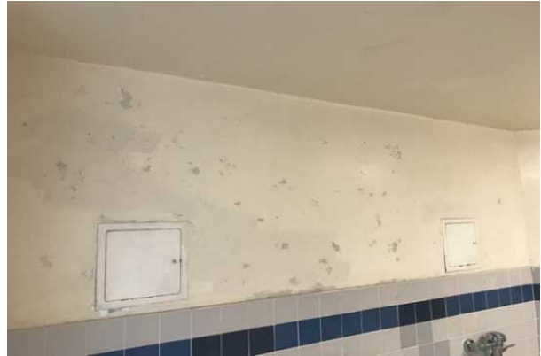
#44 CHIPPED PAINT IN RESTROOMS
