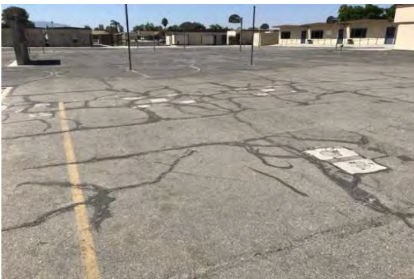
#35 CRACKED SPORTS COURTS
