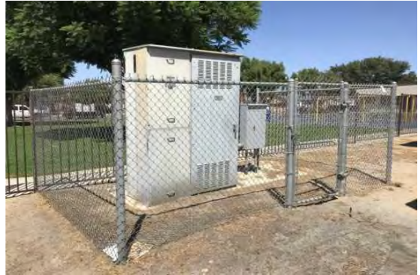
#8 PRIMARY ELECTRICAL - PORTABLE CLASSROOM
