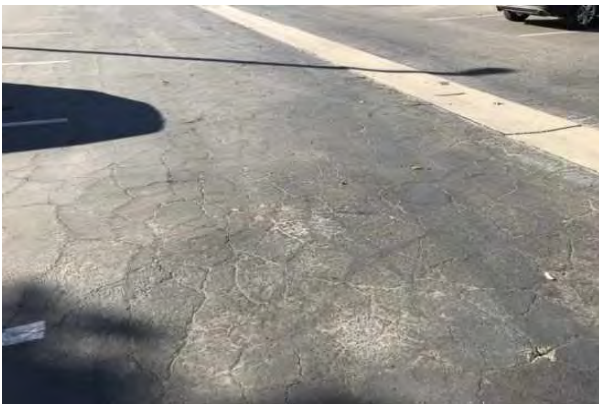
#33 CRACK ASPHALT PAVEMENT
