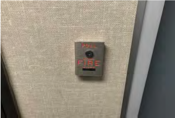
#19 FIRE ALARM SYSTEM
