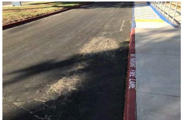
#34 CRACK ASPHALT PAVEMENT
