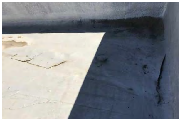
#36 DAMAGED ROOF MEMBRANE
