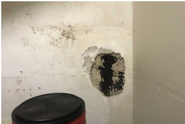
#47 DAMAGED UTILITY WALLS
