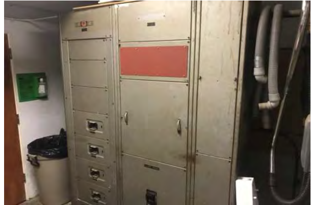
#32 MAIN ELECTRICAL EQUIPMENT
