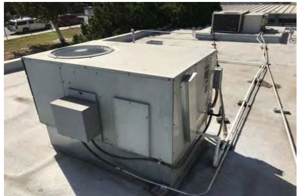
#30 MAIN BUILDINGS HVAC
