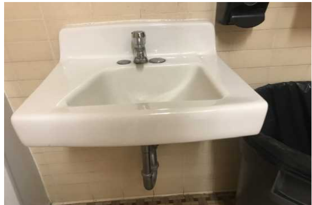
#48 LAVATORIES LACK PIPE WRAPPING
