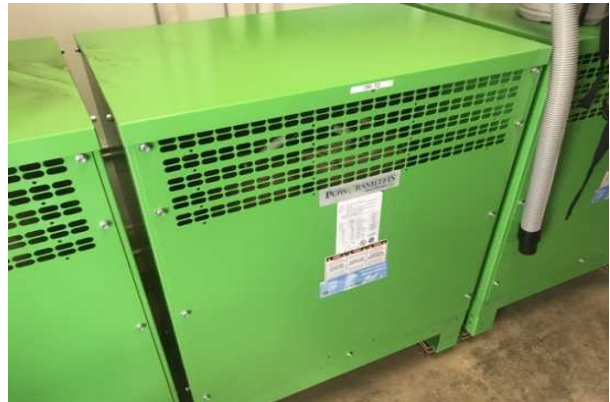
#34 NEW ELECTRICAL EQUIPMENT
