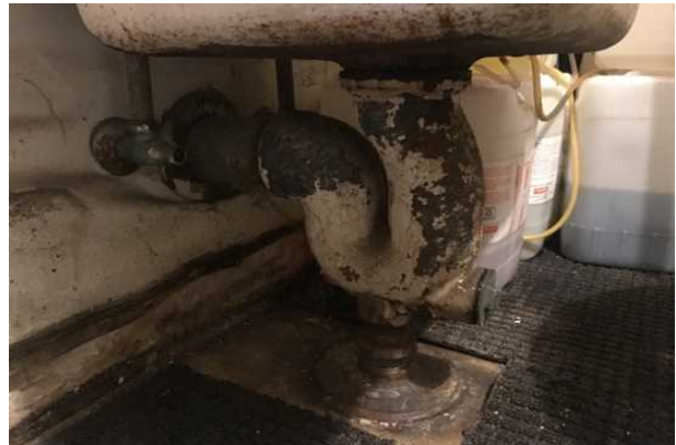
#46 SEWAGE PIPING, PRONE TO BACK-UPS
