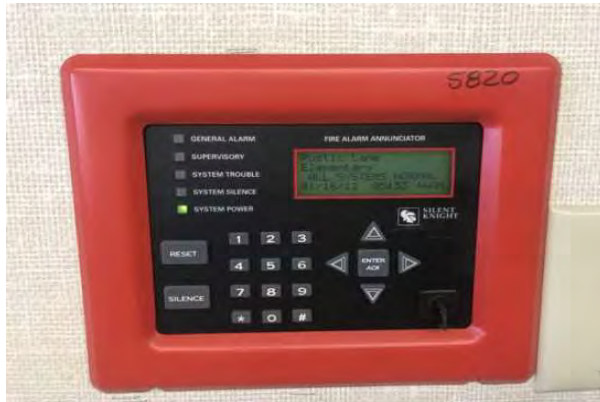
#39 FIRE ALARMS SYSTEM
