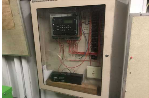
#38 FIRE ALARM CONTROL PANEL
