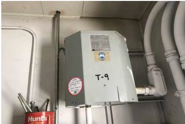
#33 SECONDARY ELECTRICAL EQUIPMENT
