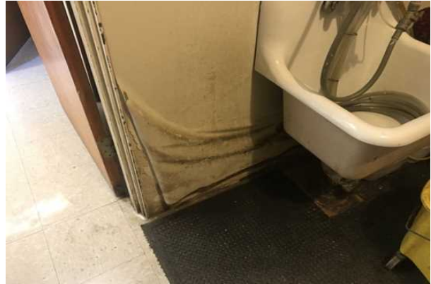
#44 DAMAGED VINYL WALLS
