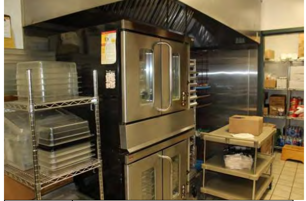
#50 COMMERCIAL KITCHEN, CONVECTION OVEN, DOUBLE
