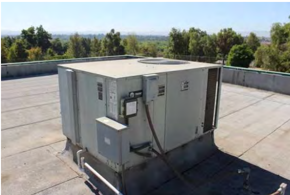
#35 PACKAGED UNIT (RTU)
