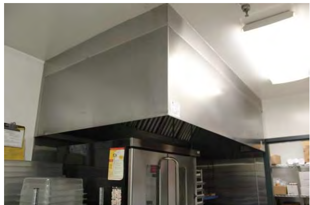
#48 COMMERCIAL KITCHEN, EXHAUST HOOD
