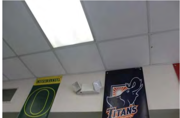
#44 EMERGENCY LIGHT, 2-HEAD WITH BATTERY
