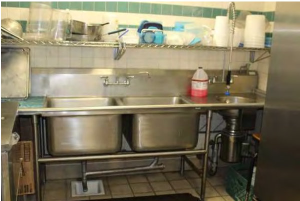
#27 COMMERCIAL KITCHEN SINK, STAINLESS STEEL
