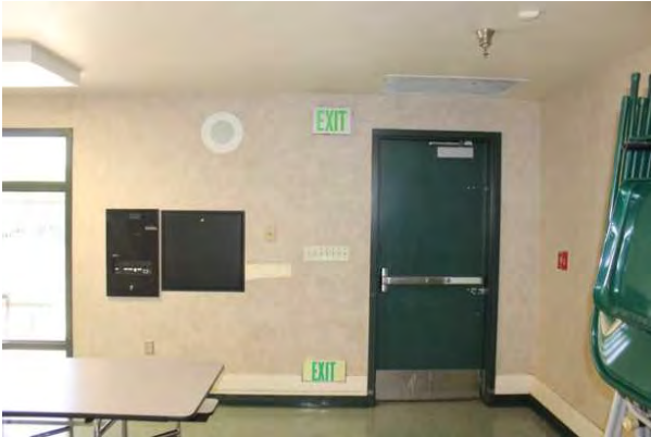
#43 EXIT SIGN LIGHT FIXTURE, LED
