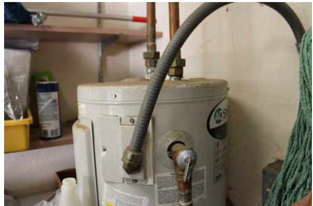
#30 WATER HEATER, ELECTRIC
