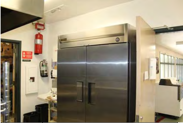
#49 COMMERCIAL KITCHEN, FREEZER, 2-DOOR REACH-IN
