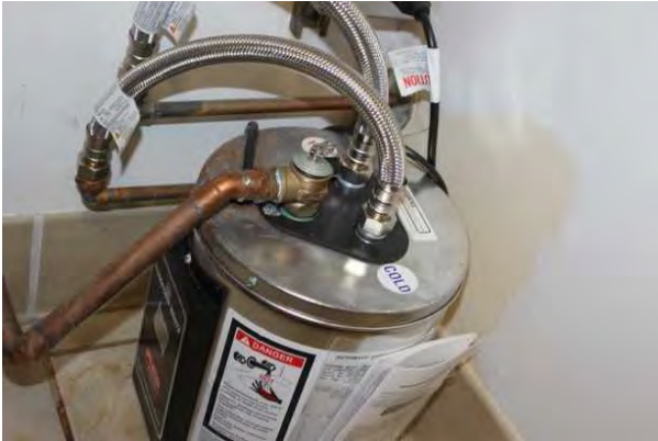
#31 WATER HEATER, ELECTRIC
