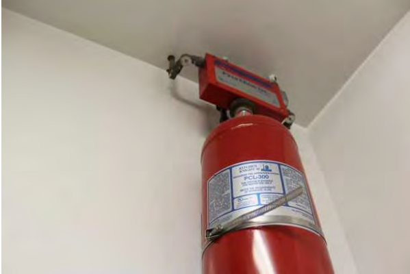
#37 FIRE SUPPRESSION SYSTEM, COMMERCIAL KITCHEN
