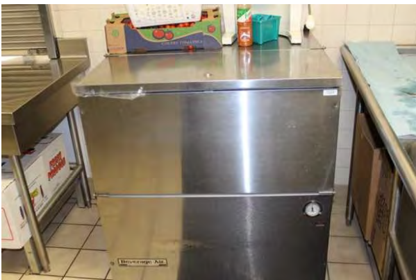
#47 COMMERCIAL KITCHEN, FREEZER, CHEST
