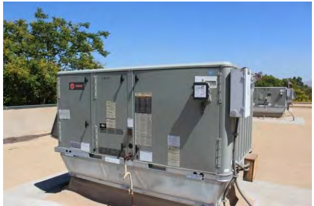
#34 PACKAGED UNIT (RTU)
