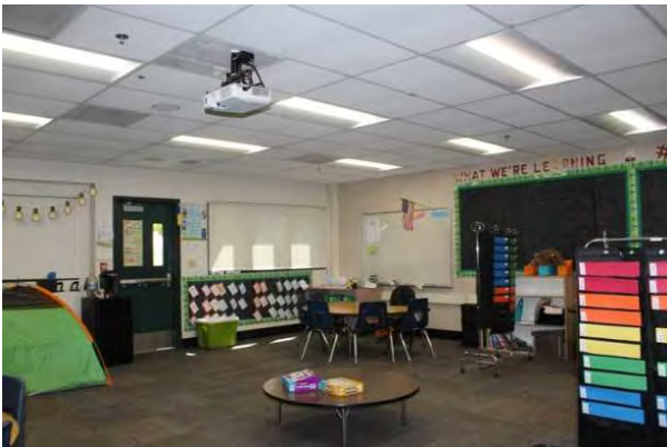
#41 LIGHTING SYSTEM, INTERIOR
