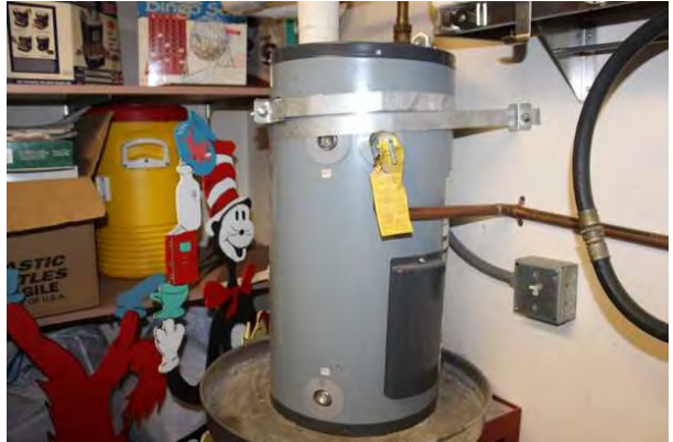
#32 WATER HEATER, ELECTRIC
