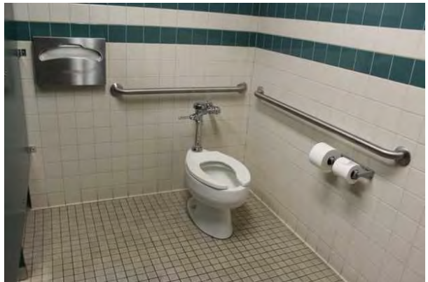
#24 TOILET, COMMERCIAL WATER CLOSET
