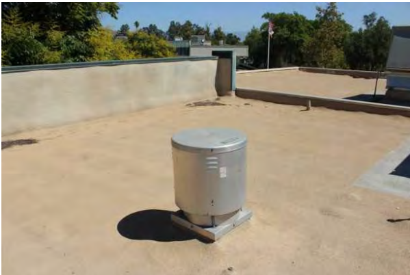
#33 EXHAUST FAN, ROOF
