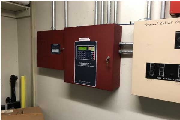
#33 FIRE ALARM CONTROL PANEL
