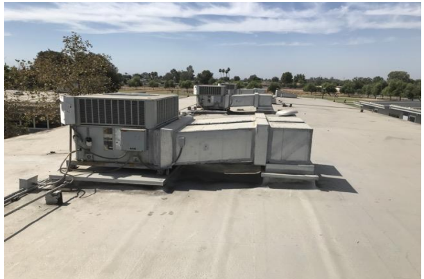
#28 CLASSROOMS BUILDINGS ROOFTOP PACKAGED UNIT
