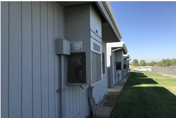
#29 PORTABLE CLASSROOMS HEAT PUMPS
