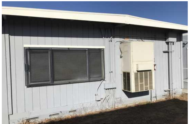
#30 PORTABLE CLASSROOMS HEAT PUMP
