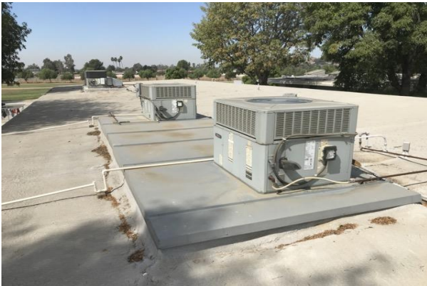
#27 CLASSROOMS BUILDINGS ROOFTOP PACKAGED UNIT
