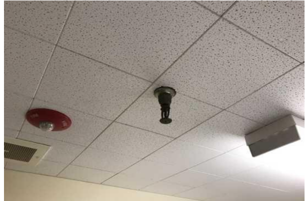
#38 FIRE STROBE/ HORN COMBO, FIRE SPRINKLER HEAD
