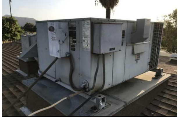
#26 ROOFTOP PACKAGE UNIT
