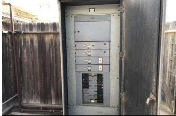
#32 EXTERIOR ELECTRICAL PANEL
