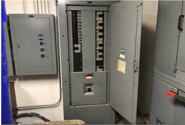
#31 INTERIOR ELECTRICAL PANEL
