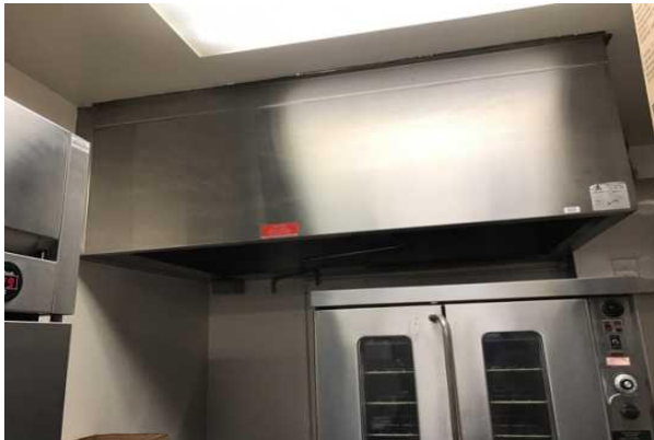
#45 KITCHEN EXHAUST HOOD
