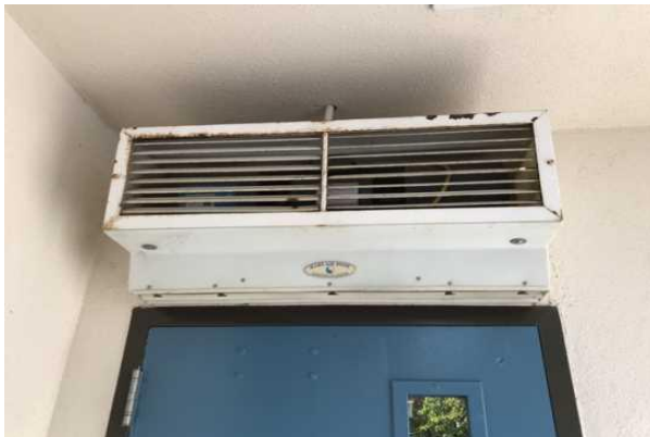
#29 AIR CURTAIN UNIT
