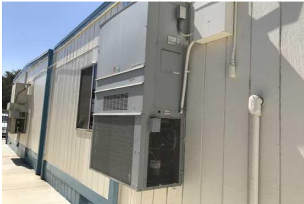
#27 WALL MOUNTED HEAT PUMP
