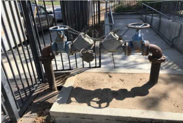
#49 SITE BACKFLOW PREVENTER
