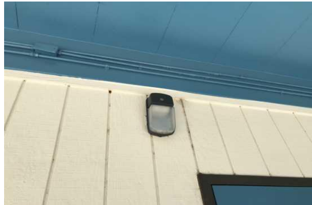
#34 EXTERIOR BUILDING METAL HALIDE FIXTURE
