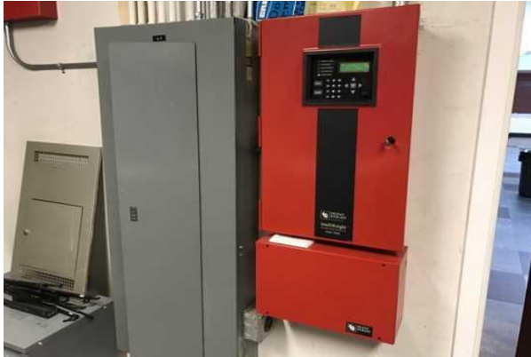
#37 FIRE CONTROL PANEL
