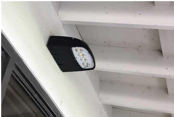
#35 EXTERIOR LED LIGHT FIXTURE
