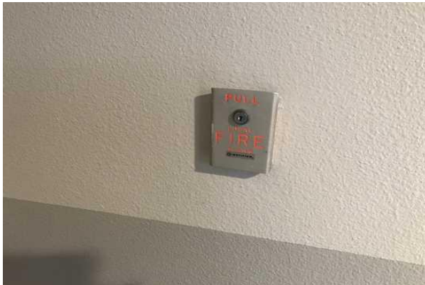
#39 FIRE PULL STATION
