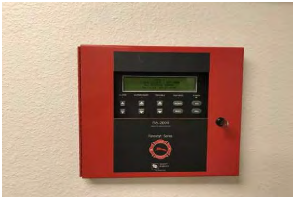
#11 FIRE ALARM PANEL
