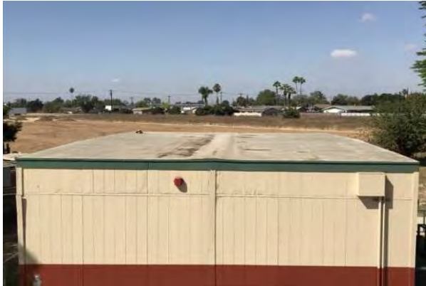
#25 DEFICIENCY - ROOF LEAK
