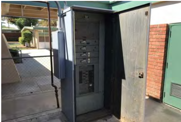
#27 DEFICIENCY - OUT OF SERVICE SWITCHBOARD
