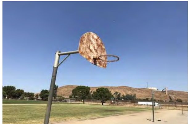
#30 DEFICIENCY - RUSTED BASKETBALL BACKBOARD
