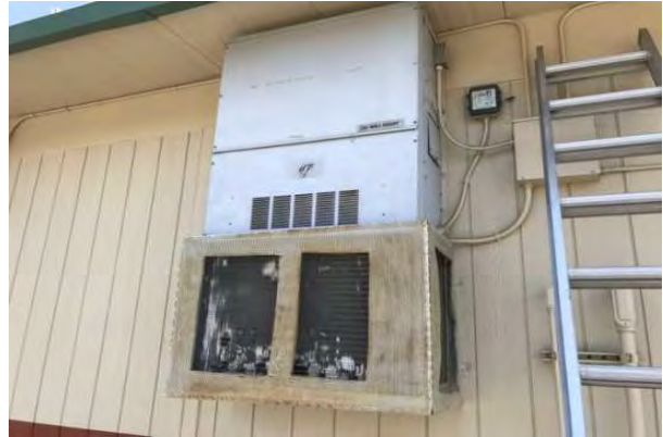
#26 DEFICIENCY - WALL MOUNTED HEAT PUMP UNIT
