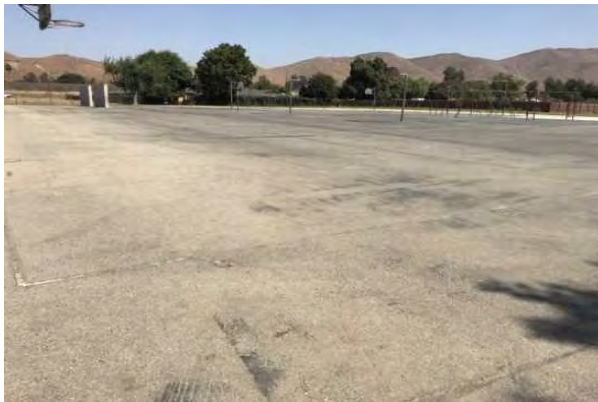
#29 DEFICIENCY - SPORTS COURTS FADED STRIPPING
