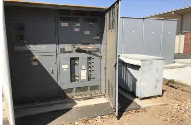
#8 EXISTING PRIMARY SWITCHBOARD
