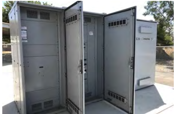
#10 NEW PRIMARY SWITCHBOARD
