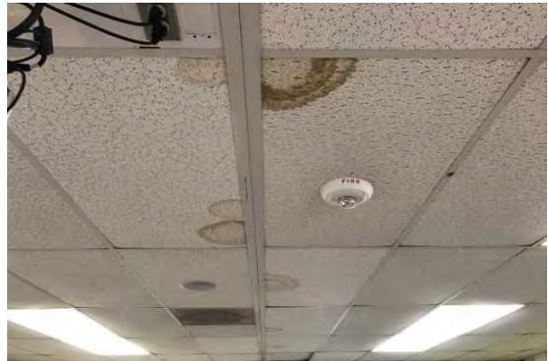
#28 DEFICIENCY - ROOF LEAK
