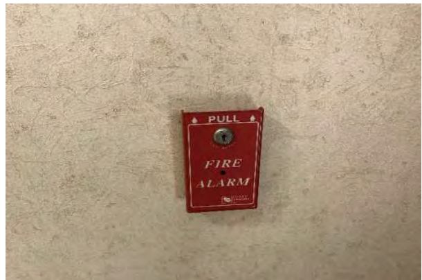
#36 FIRE PULL STATION
