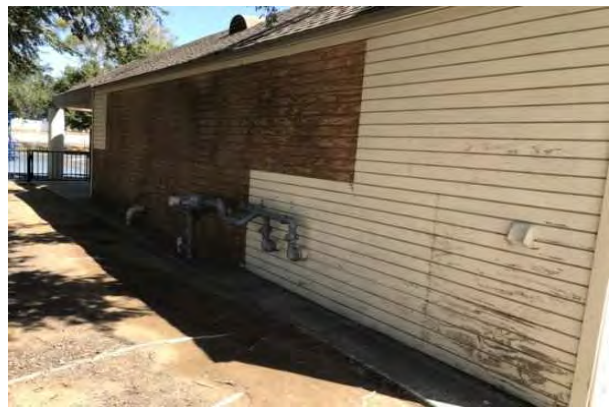
#46 PEELING AND CRACKING EXTERIOR WOOD FACADE
