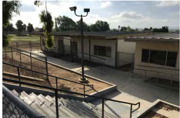
#32 SITE POLE LIGHT FIXTURE, EXTERIOR CONCRETE STAIR
