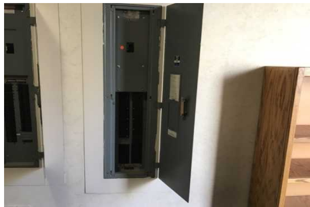
#28 INDOOR ELECTRICAL PANEL
