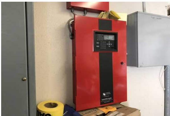
#33 FIRE CONTROL PANEL
