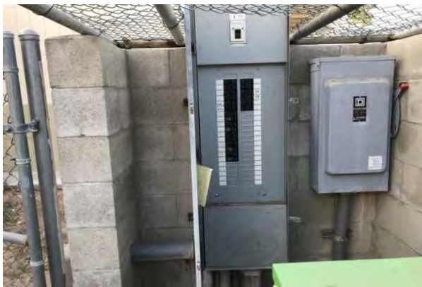
#27 OUTDOOR ELECTRICAL PANEL
