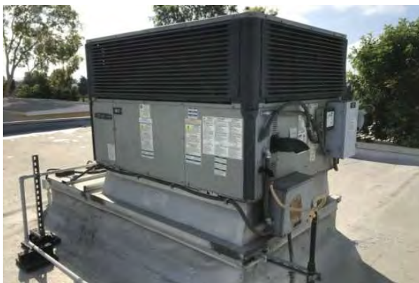
#23 ROOFTOP PACKAGE UNIT
