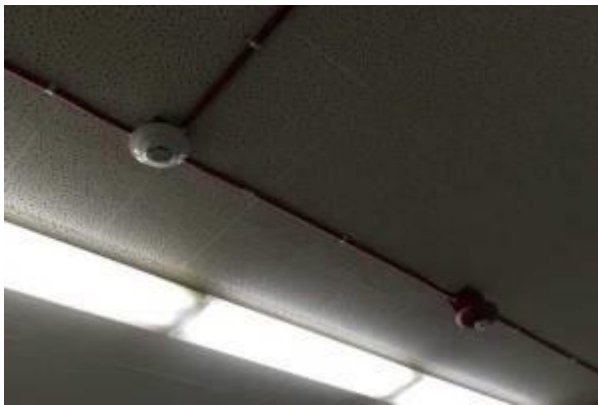
#33 LIGHTING SYSTEM, INTERIOR
