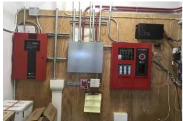
#34 FIRE ALARM CONTROL PANEL
