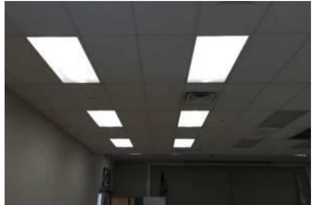
#32 LIGHTING SYSTEM, INTERIOR
