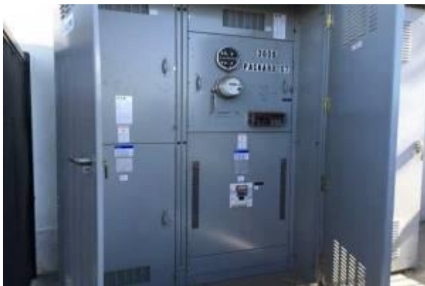
#29 MAIN DISTRIBUTION PANEL
