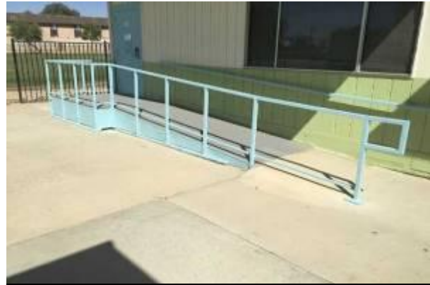
#14 EXTERIOR STAIR/RAMP RAILS, WOOD, REFINISH
