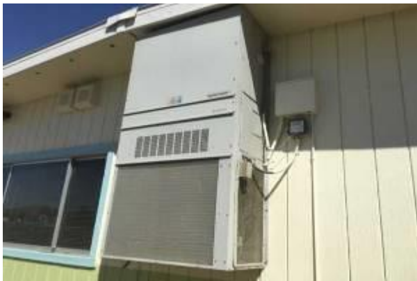
#27 HVAC WALL UNIT
