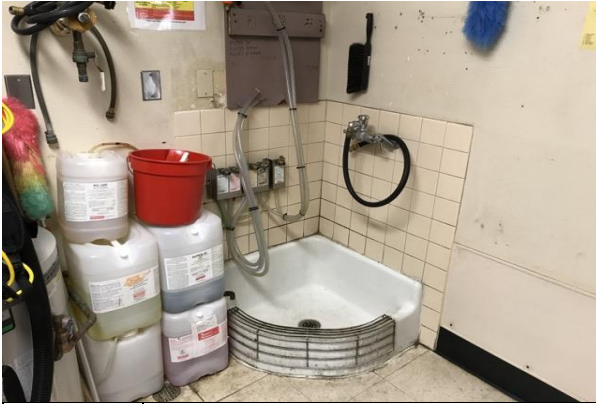
#25 FLOOR SERVICE SINK
