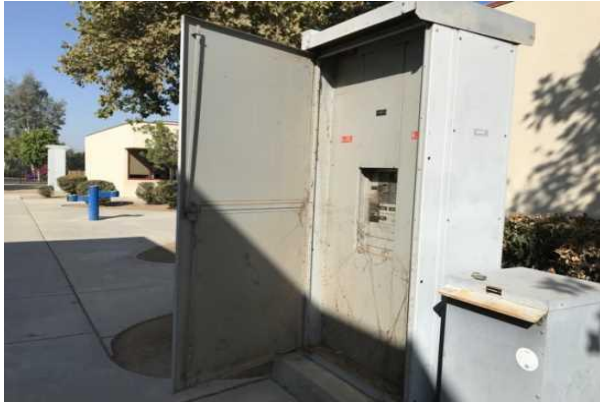
#31 EXTERIOR ELECTRICAL PANEL
