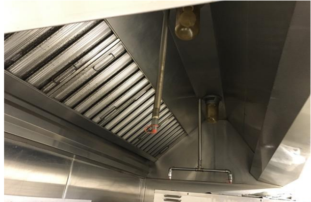
#38 KITCHEN HOOD FIRE SUPPRESSION SYSTEM
