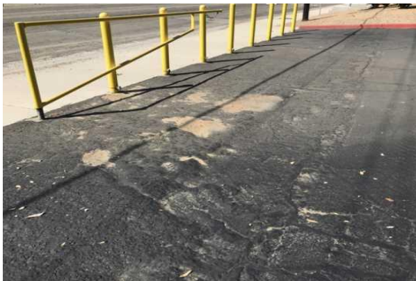
#51 DAMAGED ASPHALT SURFACE
