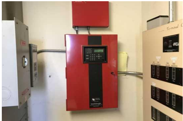
#36 FIRE CONTROL PANEL
