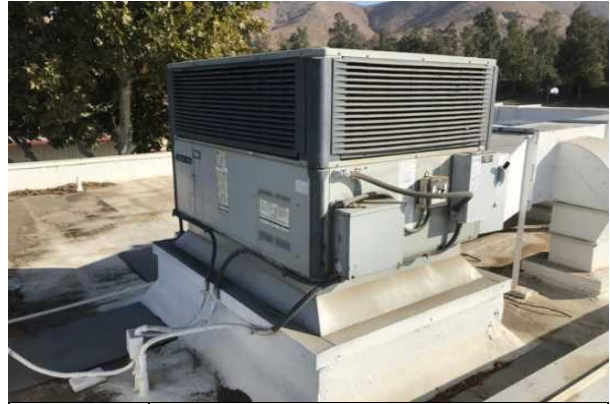
#26 ROOFTOP PACKAGE UNIT
