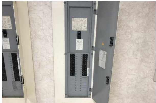
#30 INTERIOR ELECTRICAL PANEL
