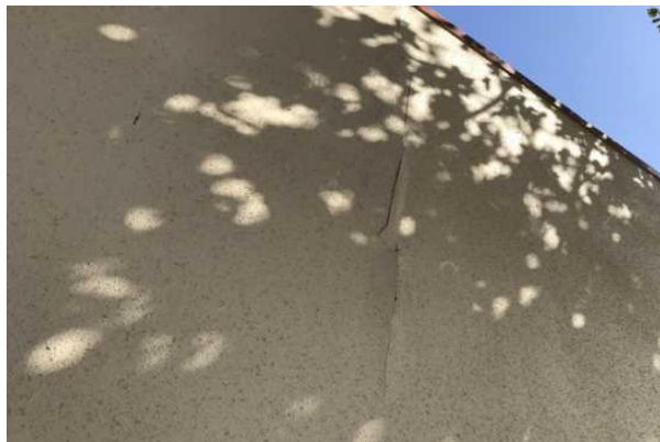
#15 DAMAGED EXTERIOR STUCCO FACADE
