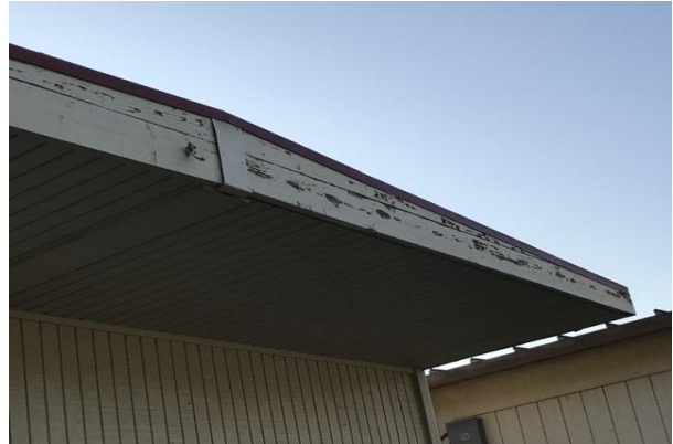
#50 PEELING AND CRACKING WOOD TRIMMING
