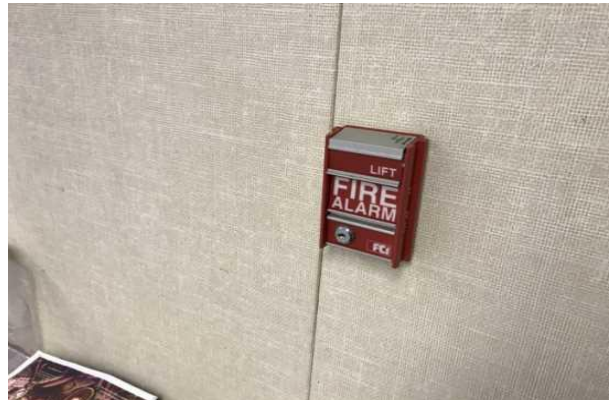
#40 FIRE PULL STATION
