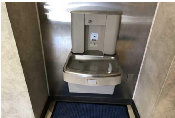
#23 INTERIOR DRINKING FOUNTAIN
