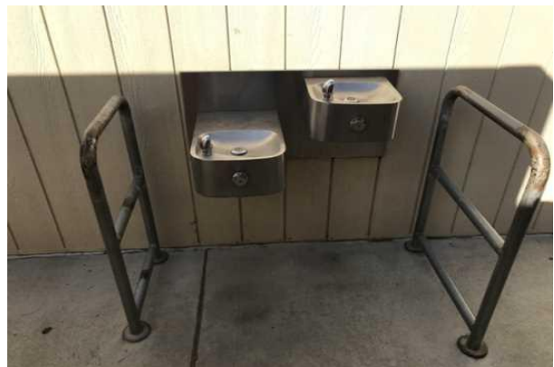
#24 OUTSIDE DRINKING FOUNTAIN
