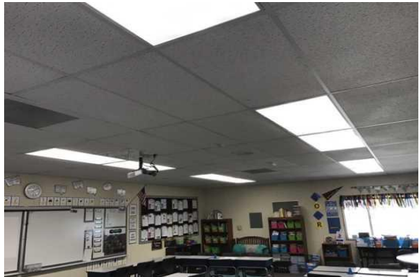
#34 INTERIOR LIGHTING SYSTEM
