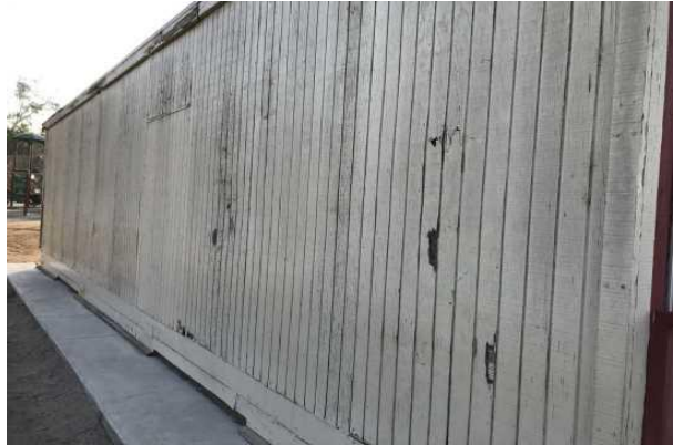
#14 DAMAGED WOOD FACADE
