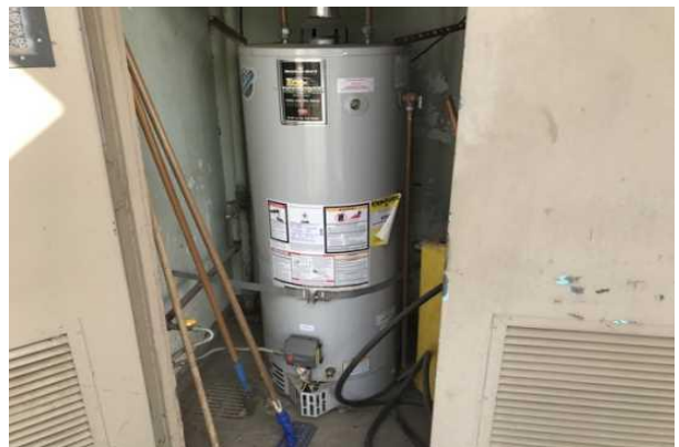
#18 MPR BUILDING - WATER HEATER
