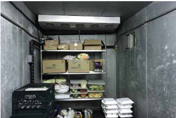
#35 MPR BUILDING KITCHEN - WALK-IN COOLER
