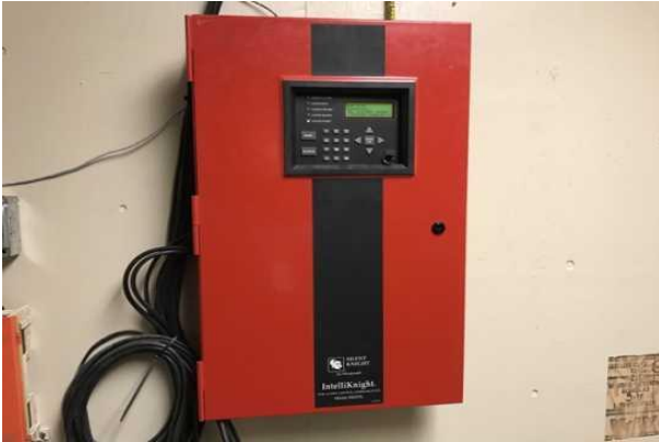
#19 FIRE ALARM PANEL
