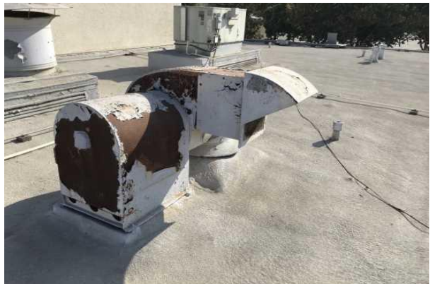
#24 MPR BUILDING - EXHAUST FAN
