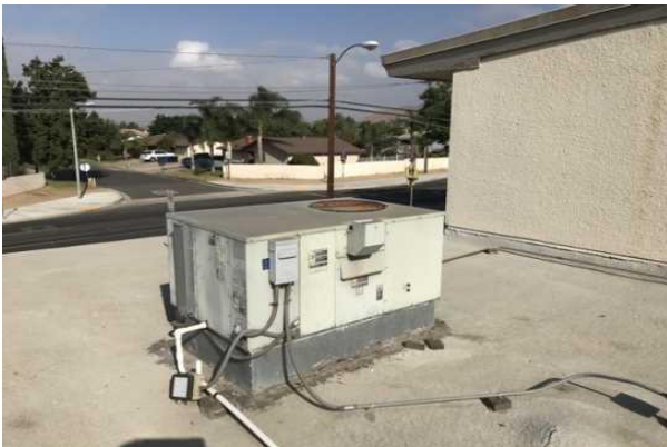
#23 MPR BUILDING - PACKAGED UNIT
