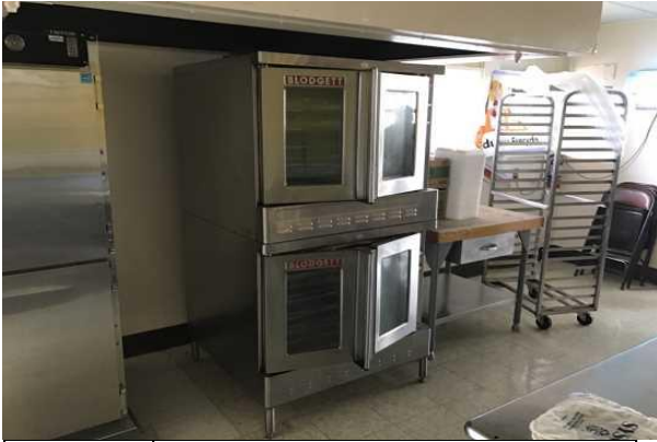
#31 MPR BUILDING KITCHEN - OVENS
