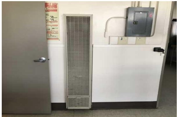
#36 MPR BUILDING KITCHEN - FURNACE
