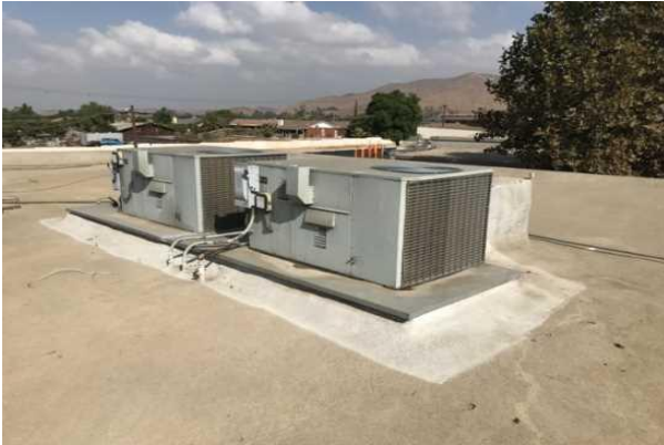
#25 CLASSROOMS BUILDING - PACKAGED UNITS
