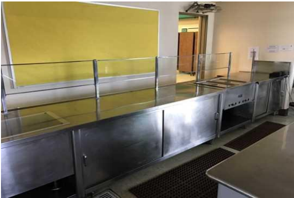
#33 MPR BUILDING KITCHEN - FOOD WARMER
