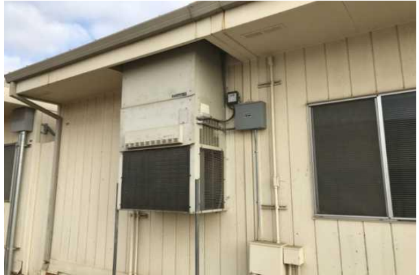
#26 PORTABLE CLASSROOMS - HEAT PUMP
