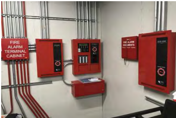
#17 FIRE ALARM PANEL
