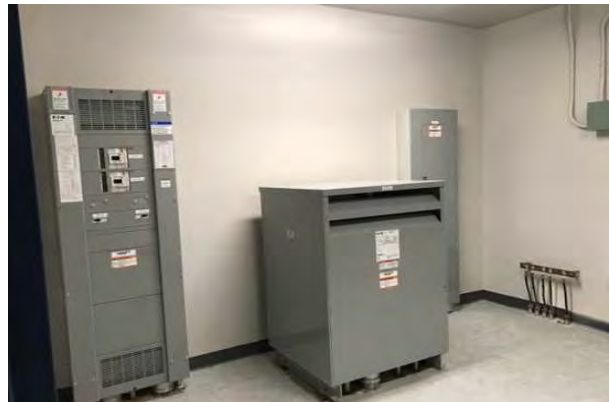
#18 ELECTRICAL ROOM - 2ND FLOOR WEST
