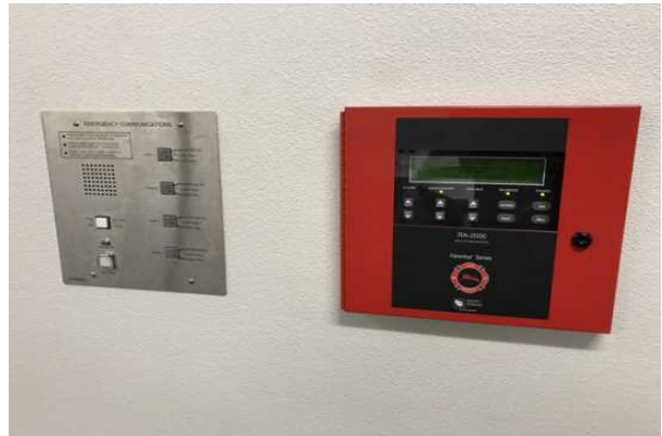
#16 FIRE ALARM PANEL
