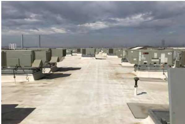
#15 HVAC COOLING AND HEATING
