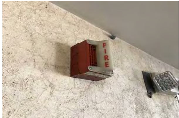
#40 FIRE STROBE/ HORN COMBO, EMERGENCY LIGHT
