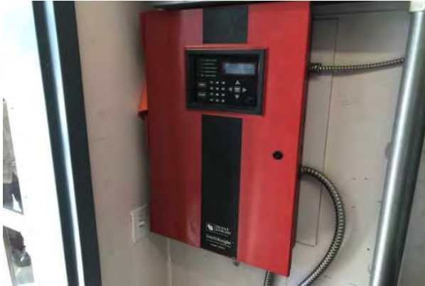
#37 FIRE CONTROL PANEL
