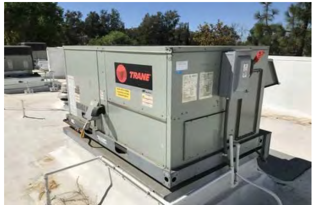
#30 ROOFTOP PACKAGING UNIT
