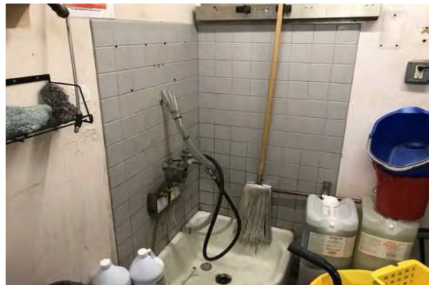
#22 FLOOR SERVICE SINK
