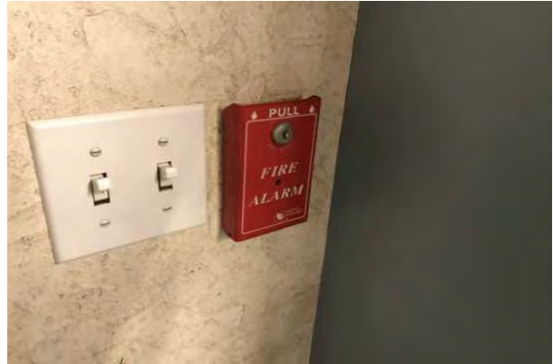
#38 FIRE PULL STATION
