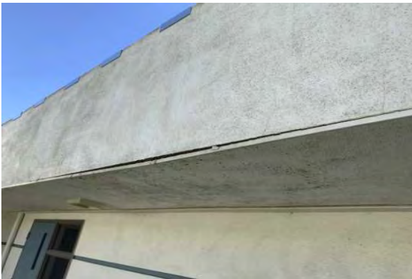
#47 WATER DAMAGED STUCCO FACADE
