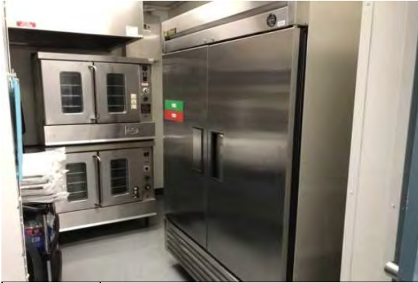
#43 2-DOOR REACH IN FREEZER, CONVECTION OVEN
