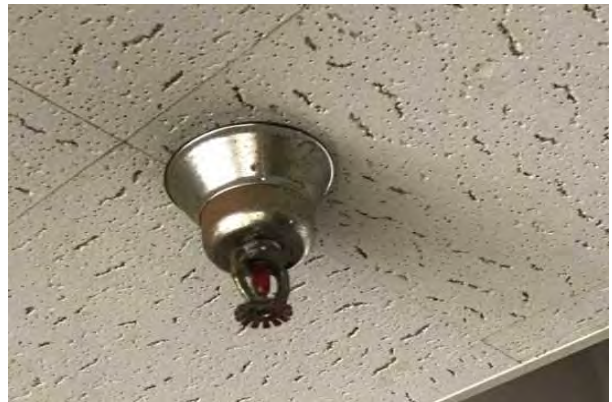
#24 MULTI-PURPOSE SPRINKLER SYSTEM
