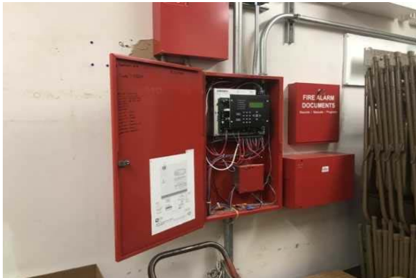
#33 FIRE ALARM CONTROL PANEL
