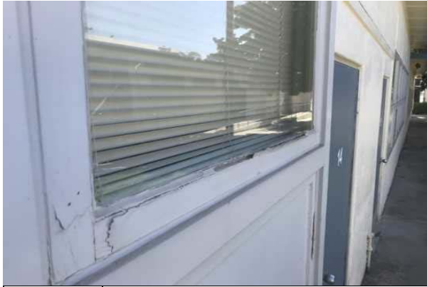
#19 DETERIORATED WOOD WINDOW FRAME AND GLAZING PUTTY
