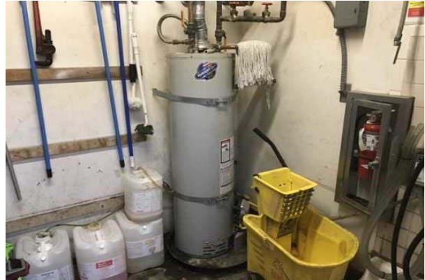
#26 DOMESTIC WATER HEATER
