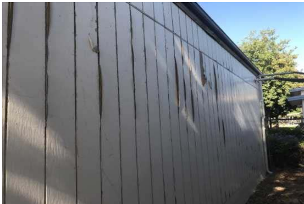
#17 DETERIORATED WOOD SIDING
