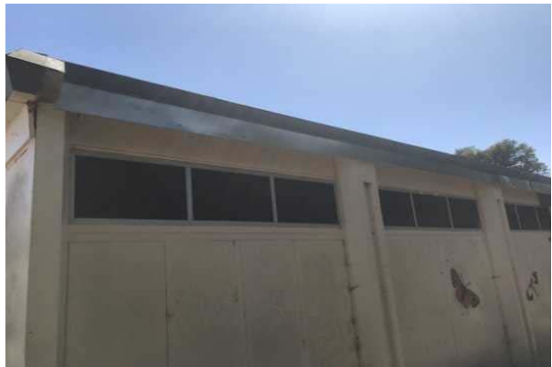
#24 DAMAGED GUTTER AND DOWNSPOUT
