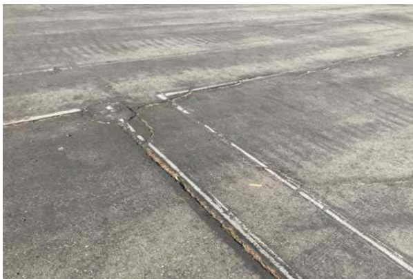
#41 DETERIORATED ASPHALT SPORTS COURT
