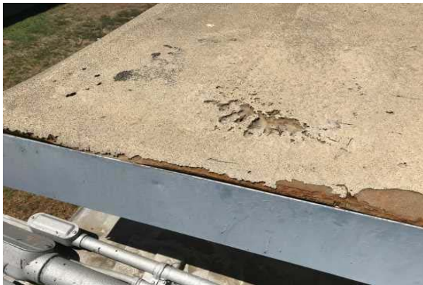
#23 DAMAGED SPRAY POLYURETHANE FOAM ROOFING
