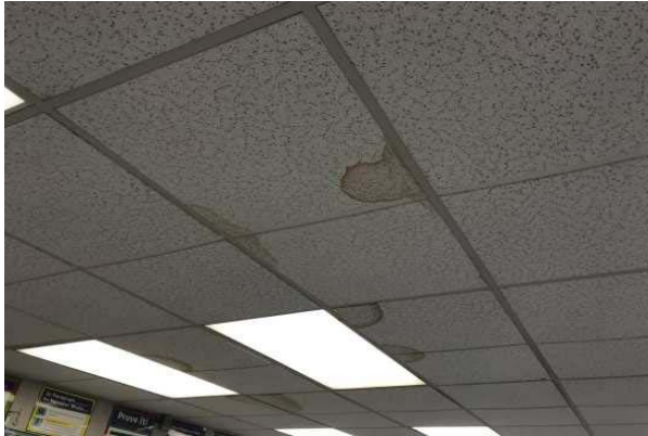
#25 STAINED CEILING TILES FROM ACTIVE ROOF LEAKS
