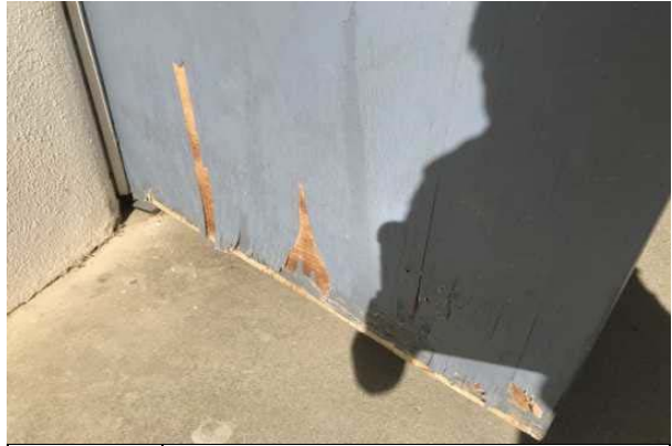
#20 DETERIORATED WOOD DOOR
