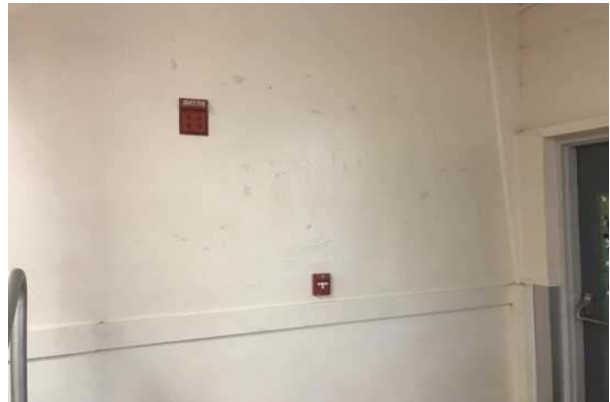
#34 FIRE ALARM SYSTEM
