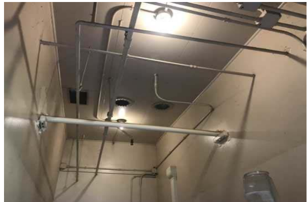
#30 PARTIAL SPRINKLER SYSTEM IN STORAGE CLOSET
