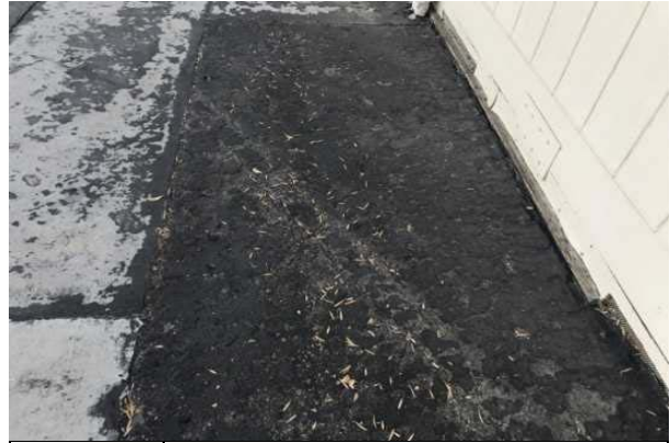
#38 WEATHERED ASPHALT WALKWAY
