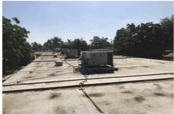
#28 ROOFTOP HVAC EQUIPMENT
